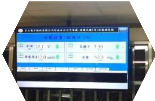
Waste water automatic connection monitoring System
