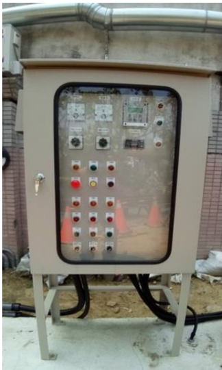
Discharge monitoring and control panel
