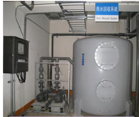
↑ Factories installed with rainwater recycling system
