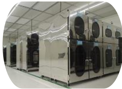
Commodity racks are fixed to resist earthquakes
