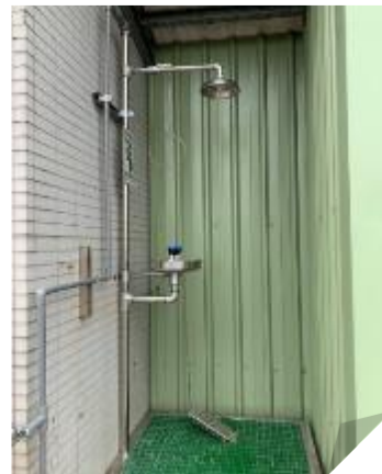
Emergency shower equipment in water treatment areas
