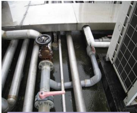
↑ Factory Rain water recycling system integration
